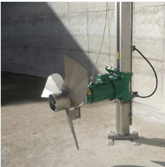
4G with EV - Closed tank
