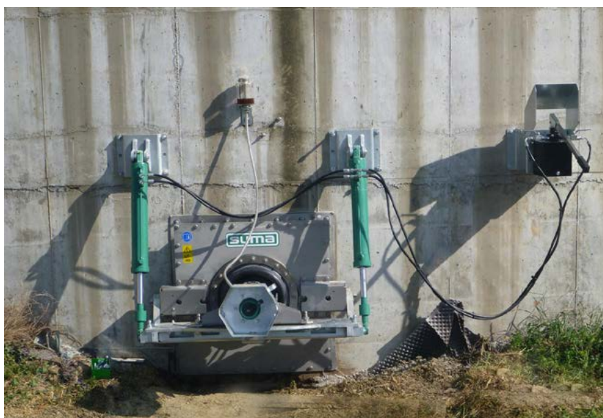
FT HY with hydraulic cylinder upwards - Concrete tank
