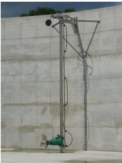
MGD - Concrete tank with 2G
