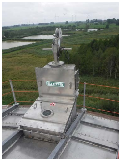
GDD - Steel tank
