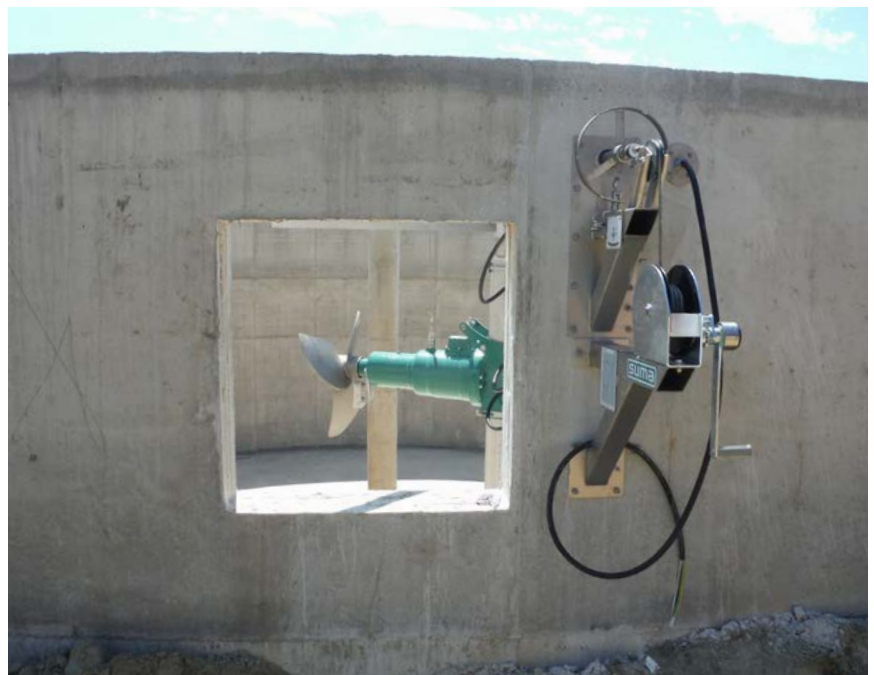
MGD - Concrete tank with 2G
