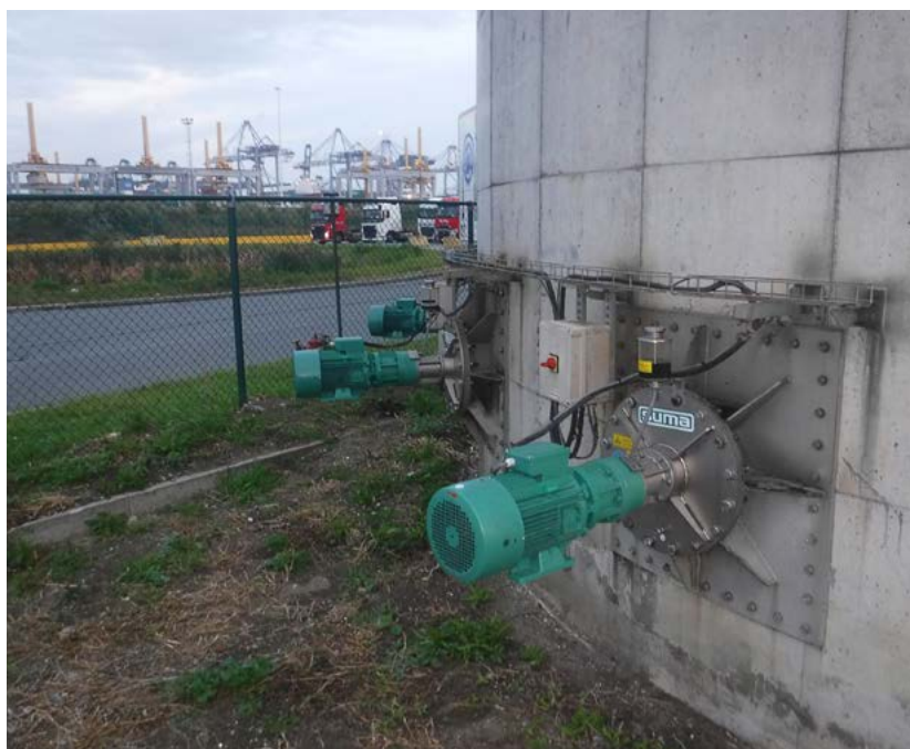
FR light - Concrete tank
