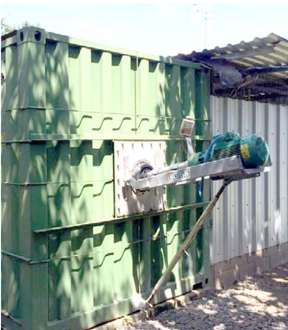
BG2 - Steel tank
